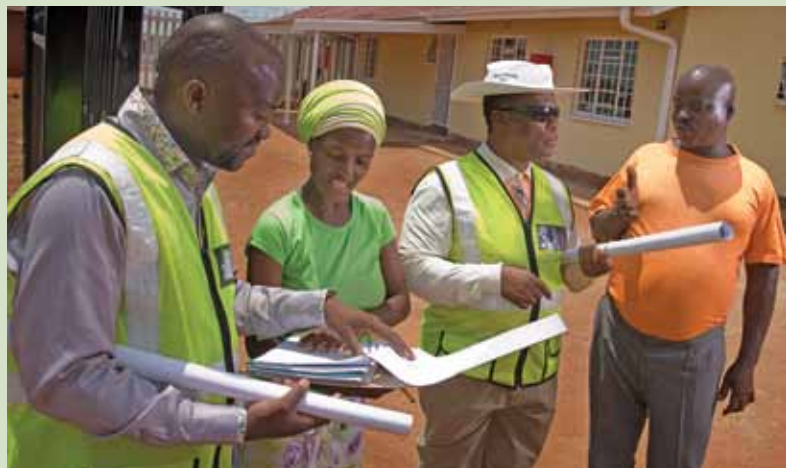
Site visit during the construction of the satellite police station and multi-purpose centre established for the benefit of the MACHARORA community
