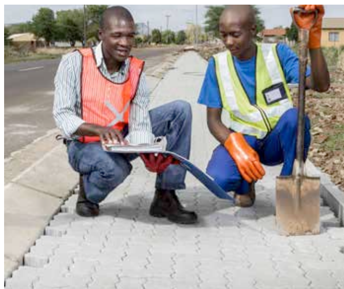
We built a pedestrian walkway in Mafenya village to keep children safe from vehicle traffic
