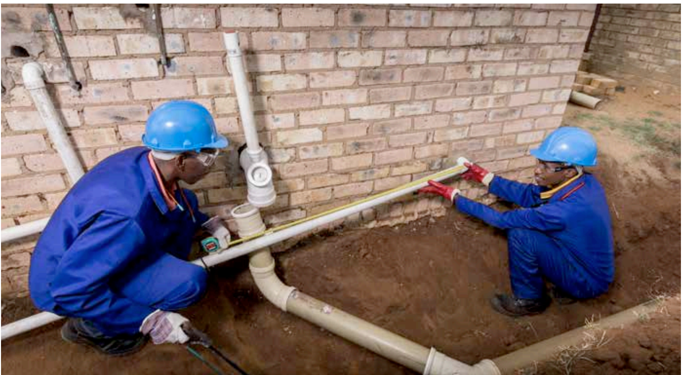
As part of BRPM's portable skills training community members are trained as plumbers
