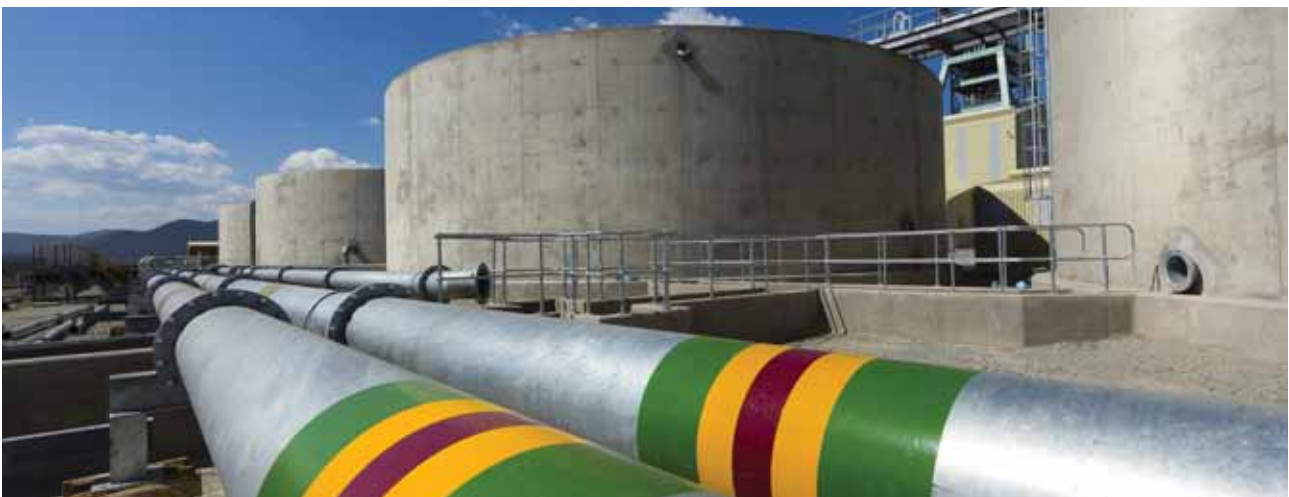
Service water infrastructure at Styldrift I
