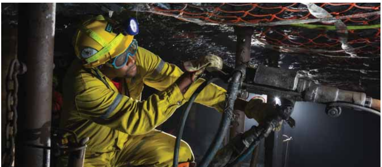
A rock drill operator working in a stoping area at our BRPM North shaft
