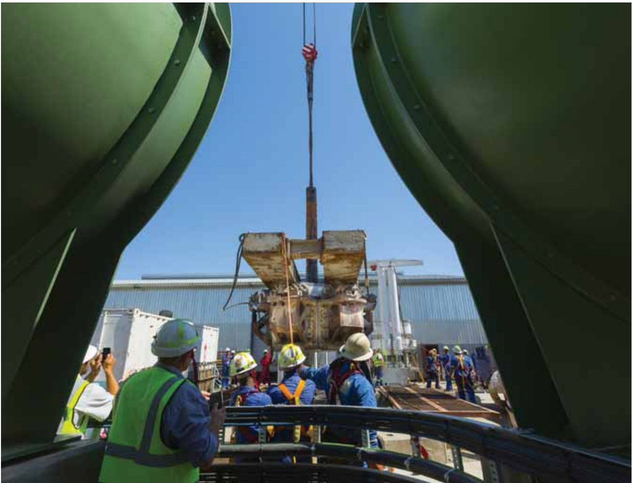
Removal of raise bore machine base after completing reaming of Ventilation shaft I
