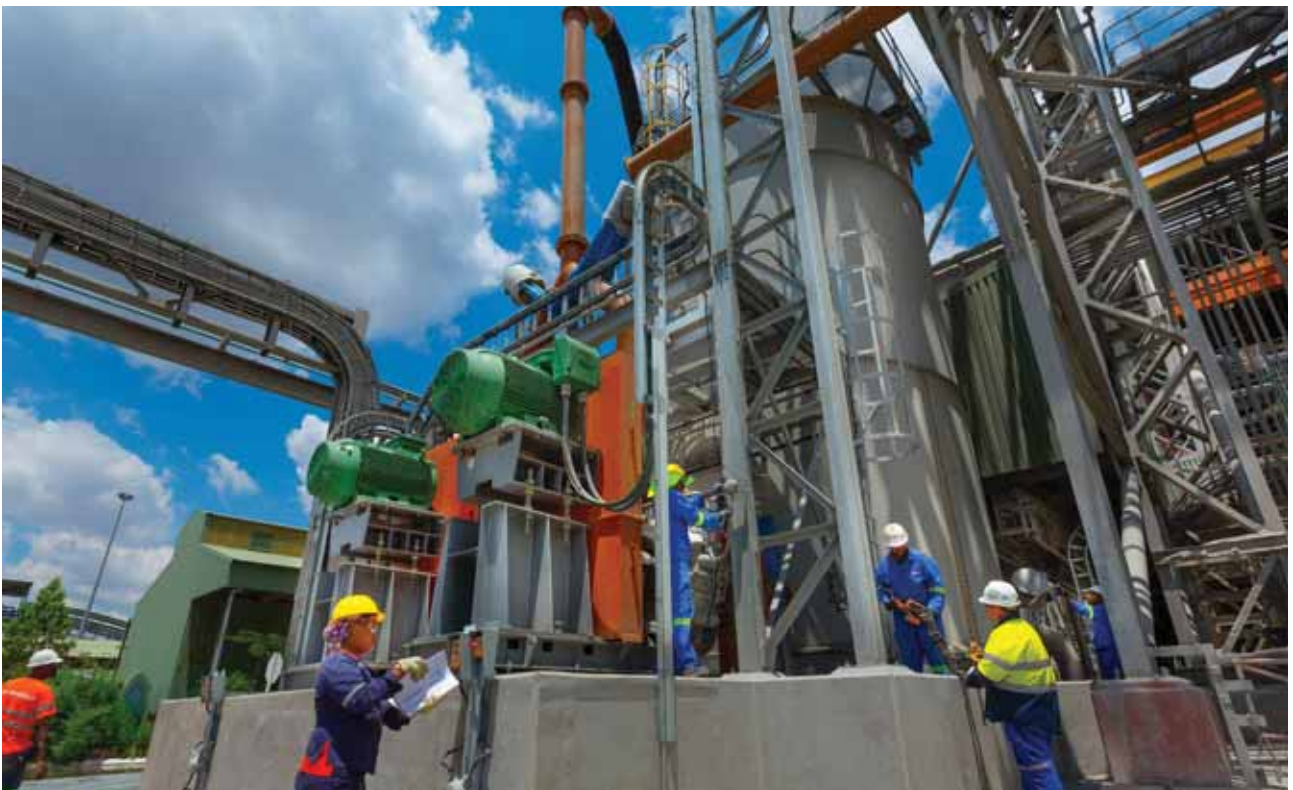
BRPM 250ktpm concentrator upgrade project, for which completion has been deferred to the first quarter of 2016
