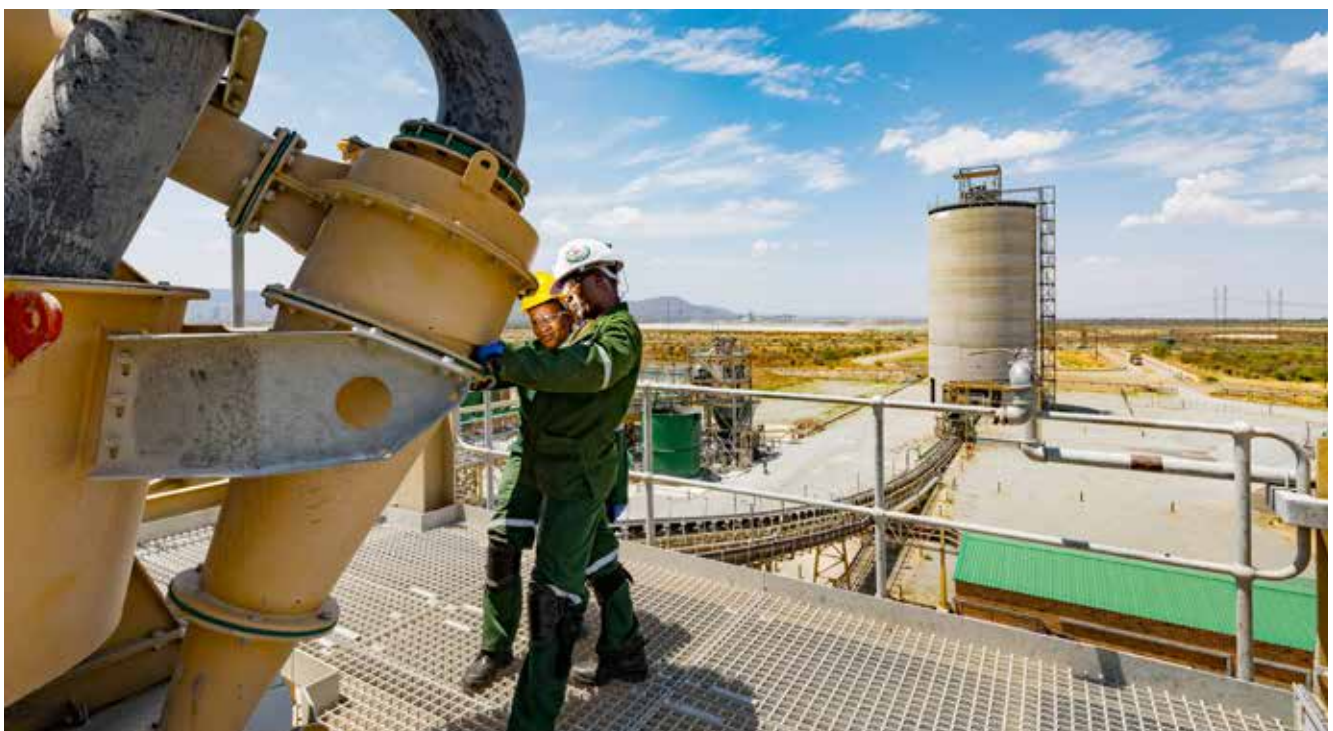
The Cyclone at the Maseve concentrator
