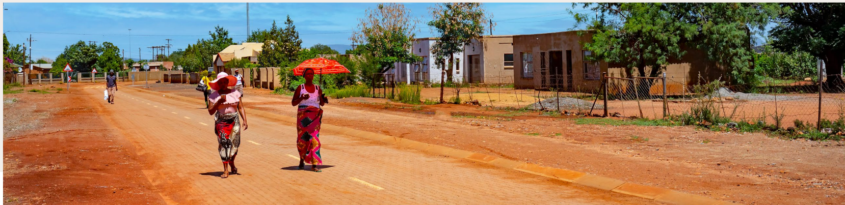
One of the new paved roads RBPlat constructed in the Macharora villages, which were the main focus of our investment in community infrastructure in 2021
