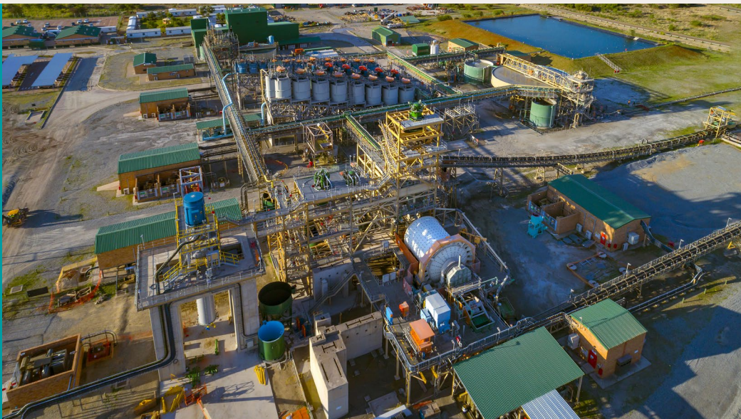
Maseve concentrator with primary ball mill and secondary H29 mill in the foreground
