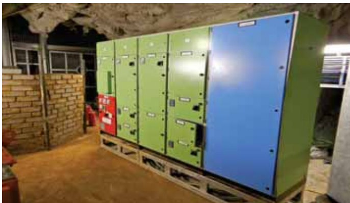
600 level - production section MCC installation
