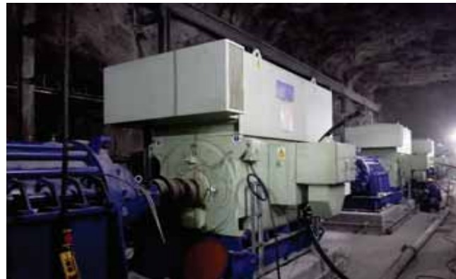
708 level - Main pump station (MPS)
